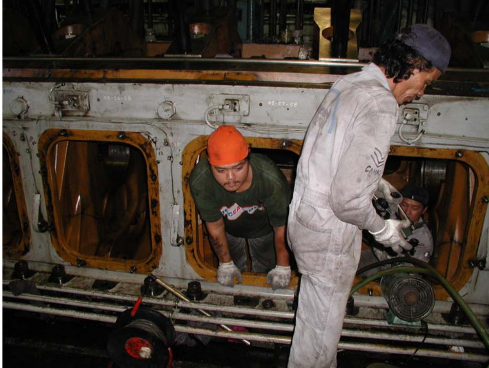
Overhaul of 13 MW Engine
